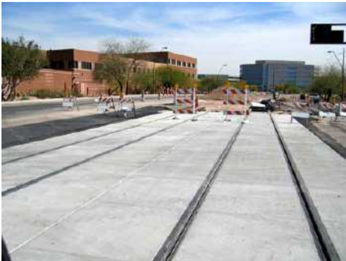
The first stretch of double track for the new METRO light rail system was laid on East Washington Street in Phoenix last month. —Marc Pearsall photo
